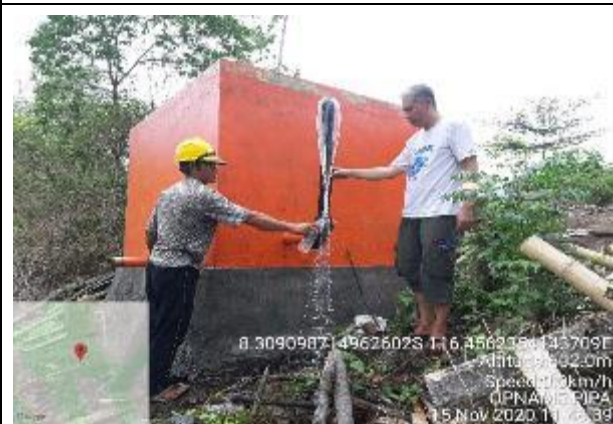
6 Clean water distribution reservoir
